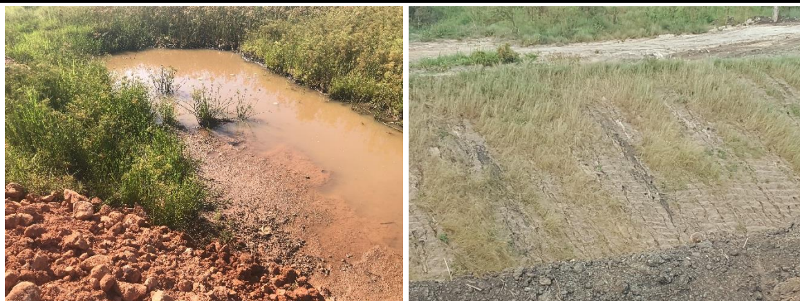
Figure 5.12 Evidence of sediment accumulation (left) and erosion gulleys within Eragrostis teff planted on embankments (right) of the SGR
